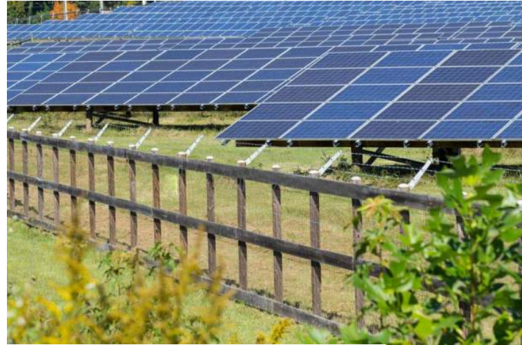
GROUND MOUNTED PV PANELS WITH FENCE
