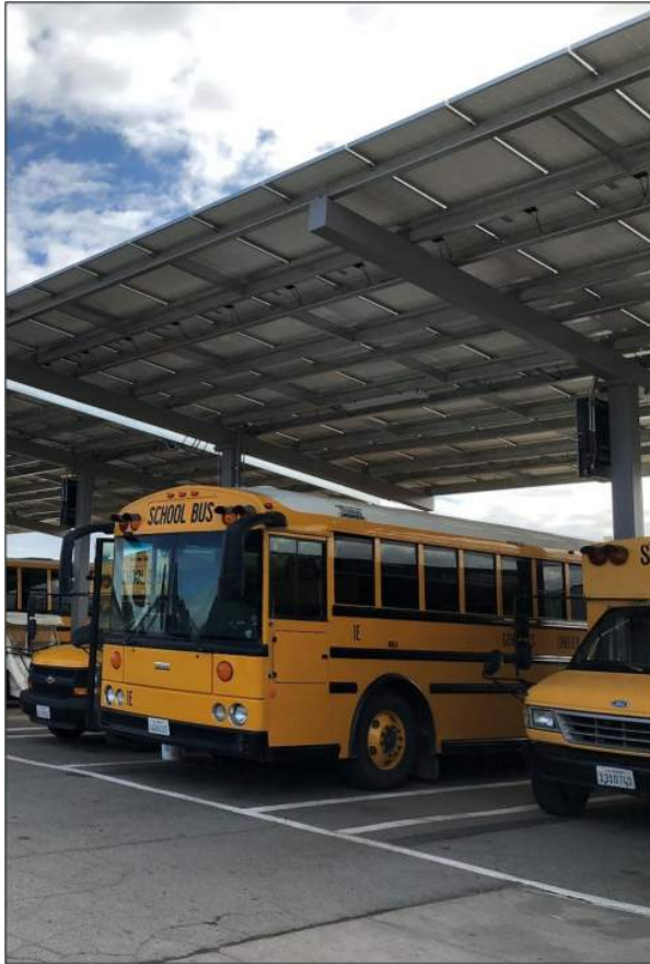
CARPORT MOUNTED PV PANELS
